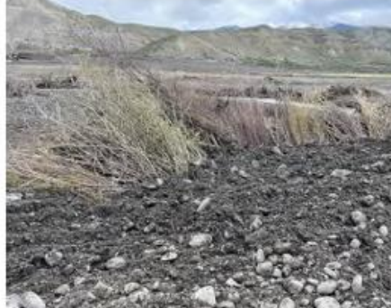
STAGE 3: TRENCH BACKFILLED WITH NATIVE ALLUVIUM AND ORGANIC TOP LAYER BEING PLACED.
