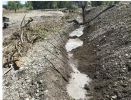
STAGE 1: MUD SLURRY IN BOTTOM OF EXCAVATED TRENCH WITH LIVE CUTTINGS PLACED.
